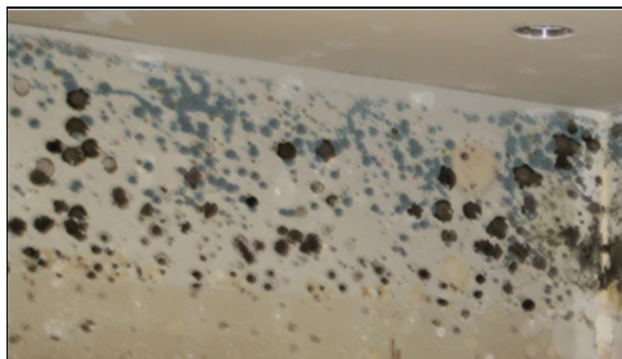
Figure 4 Mold growth on a wet wall. Here the infestation is excessive. But on your panel ceilings you may see only faint black rings – they mark the start of the process and at that stage are enough to cause product contamination
