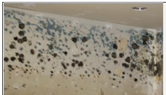
Figure 11 Mould growth on a wet wall. Here the infestation is excessive. But on your panel ceilings you may see only faint black rings – they mark the start of the process and at that stage already they are enough to cause product contamination.
