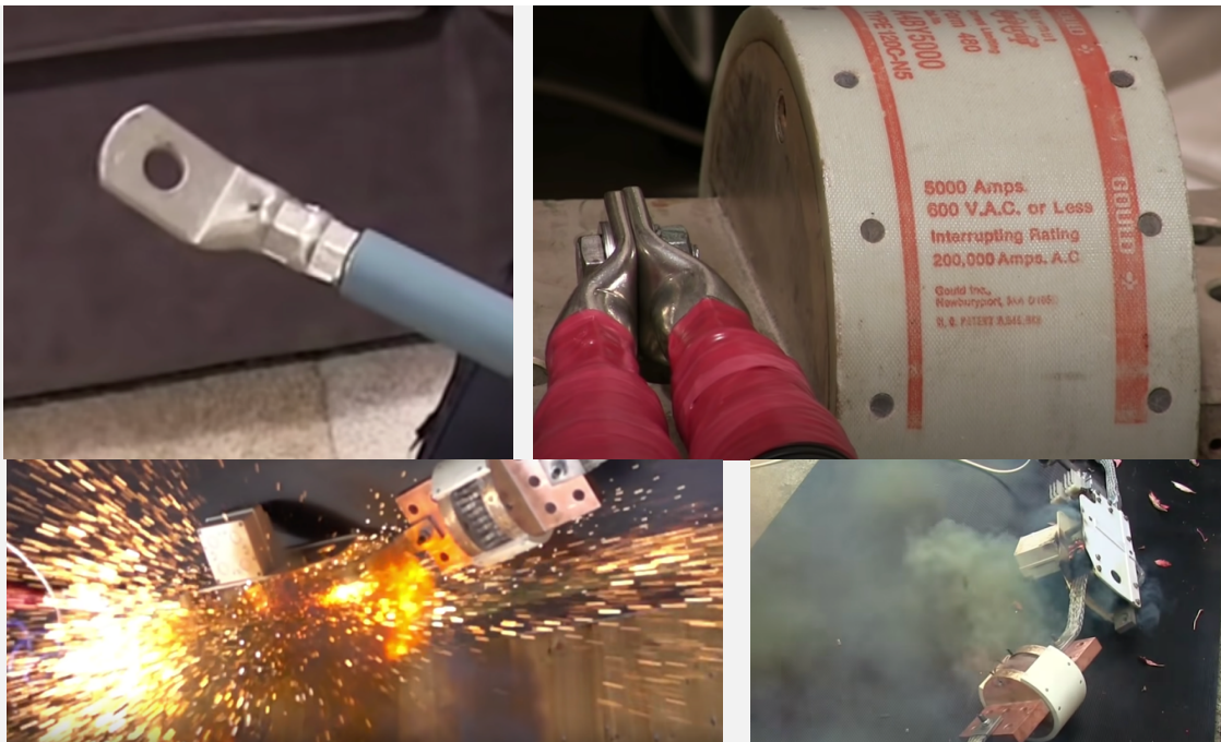
Figure 37, 38, 39, 40 Top row shows cable terminations properly crimped to ensure good conduction. When terminations are improper or when they and the cables are required to carry much higher current than they are designed for, they heat up, oxidize, which in turn further worsens the heating effect and then they reach a temperature where the metal melts or vapourizes with the effect shown in figure 39. Here some metal has vapourized or exploded and a lot of the remainder has melted into glowing sparks. In figure 40 a 5000 ampere HRC fuse has ruptured with a similar overload, but resulted in a much weaker explosion. Note the grey vapour around the fuse. It is vapourized metal. When you watch the video 36 you can experience the true magnitude of the explosions accompanying each event.
