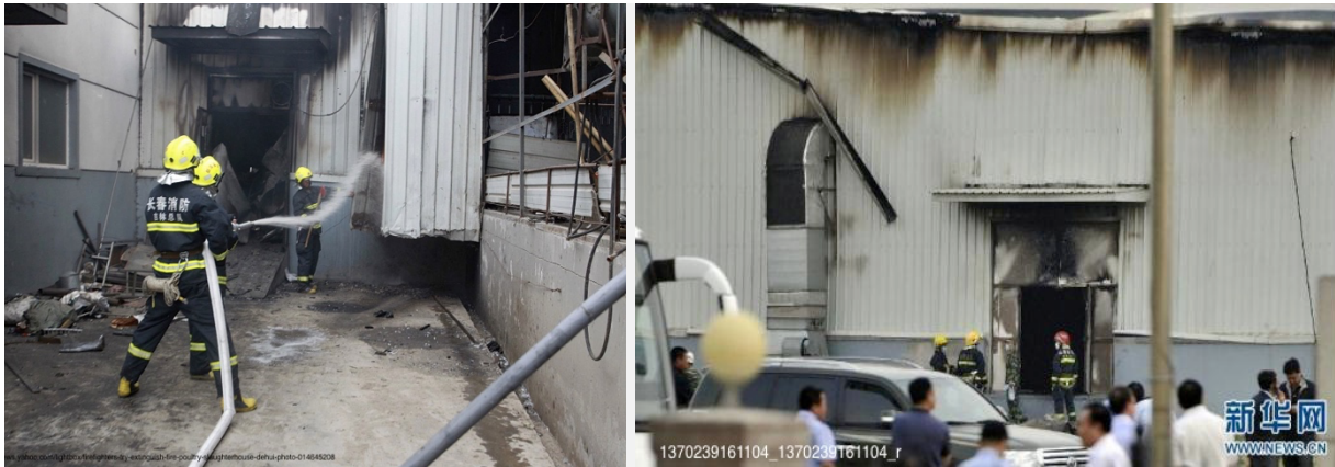
Figures 24, 25 Picture 24 (left) shows two firefighters standing in one of the lanes formed by two abutting sheds and structures to the east end of the main process building. This has been identified as a possible door between sheds 07 and 08 sheds. Note that shed 07 is intact while shed 08, which probably housed part of the rendering 2-boiler complex or the feather store, is gutted. The picture on the right (25) taken at the north side, shows some signs of fire and a collapsed roof-gutter. These form two possible emergency exits. The odd shaped door on the left was probably added as an afterthought – the height, shape and absence of protection against rain at this doorway suggesting that it opens not into the process area, but into an internally located maintenance area. 27
