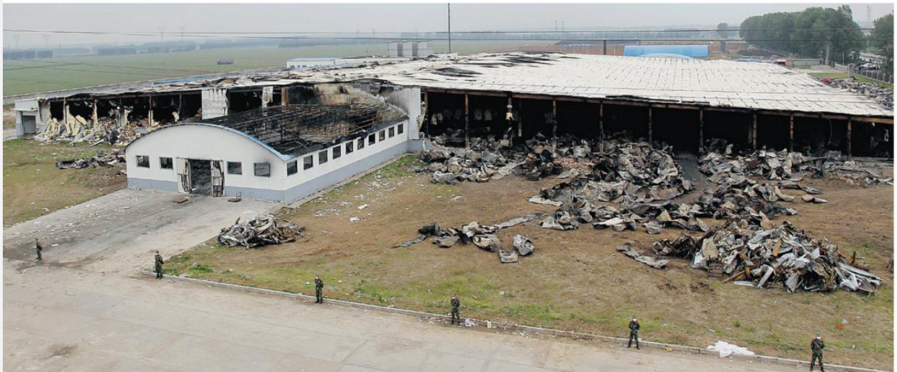
Figure 8 Aerial view of the plant after the fire had been controlled and guards were posted on its perimeter. This picture shows that the north half of the building was completely gutted, though the south half, just beyond the central ridge, remained substantially intact. Except for shed 18 in the centre and the secondary packing material receipt door (D1) on the extreme left, there were three other doors (D3, D4, D5) along the west wall, on the south of shed 18, which were destroyed as a result of rescue activities. These three doors were locked – the lawn giving ample testimony to this fact by bearing no signs of footpaths, although light traffic along the plinth protection might still have been possible. Going from left to right in the background of this picture (or along the east end), are three buildings (Buildings 01, 02 and 04), an intact smokestack arising from the vicinity of buildings 14 and 15, a truncated smokestack arising from the vicinity of sheds 08 and 09, the gable-end view of shed 08, the blue-domed Quonset hut 5 (housing the effluent treatment plant) and the gate for entry of trucks carrying live chicken. The truncated smokestack in the vicinity of sheds 09 and 08 was complete in the early stages of the fire (figure 13) and was probably deliberately cut off to allow freedom of movement to the fire engine boom.
