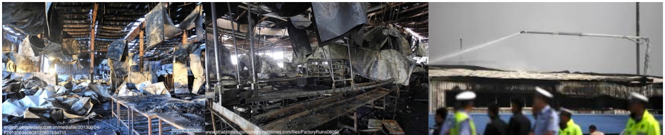
Figures 11, 12, 13 Left picture (11) shows trimming tables of a typical height of 800mm, arranged end to end. Middle picture (12) shows a J shackle line with the remains of a belt conveyor. Right picture (13) shows the presence of a second smokestack rising from somewhere in the vicinity of shed 08. The other smokestack rising from the vicinity of building 14 is also visible here.
