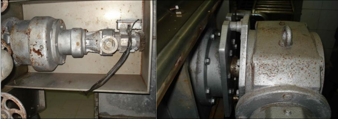
The main drive, encrusted with 28 years of paint, and closeup showing lock-pins
