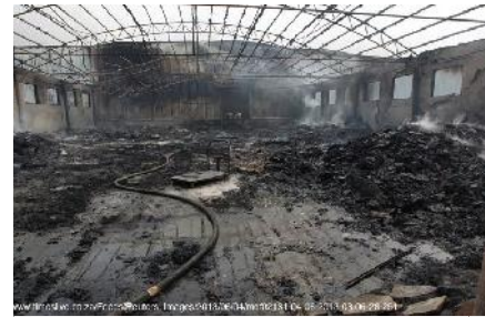
Figure 17: The burnt off roof of the finished goods dispatch shed abutting the main process shed at the West end. Note the wheeled trolley
