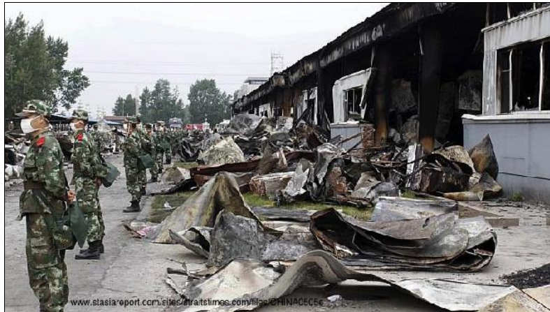
Figure 14. Taken from the East end, close to gate 2, this shows construction details. The sandwich panels in this and several other pictures have completely delaminated. Behind the main shed you can get a glimpse of the admin building and to the extreme left the row of buntings at the main gate.
