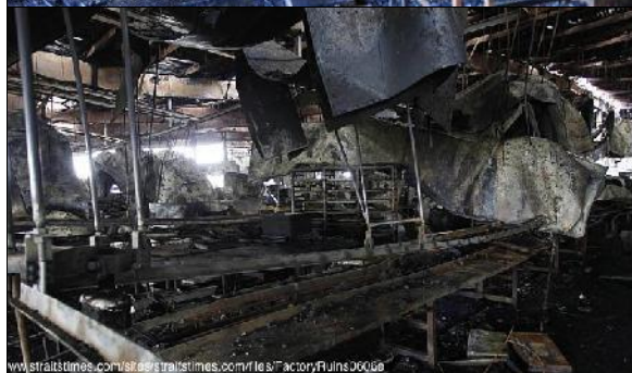
Figures 9, 10. Estimating shift capacity and probable number of workers present in the plant at the time of the fire. Top picture shows a J Shackle Stork line or its clone with the remains of a belt conveyor. Bottom picture shows trimming tables of typical height 800mm, arranged end to end. False (drop) ceiling in the bottom picture is at approximately 5-6 metres above FFL.
